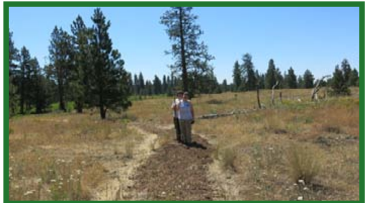
Two YCC crew members putting the finishing touches on the East Blackhorse Trail. (S. Rancourt)
